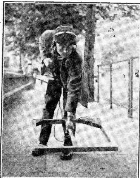
This man with the strange occupation caused passers-by to stop and stare in Trafalgar Square recently. He is an employee of the Metropolitan Water Board and was using an acoustic apparatus to trace a water main under the pavement.
