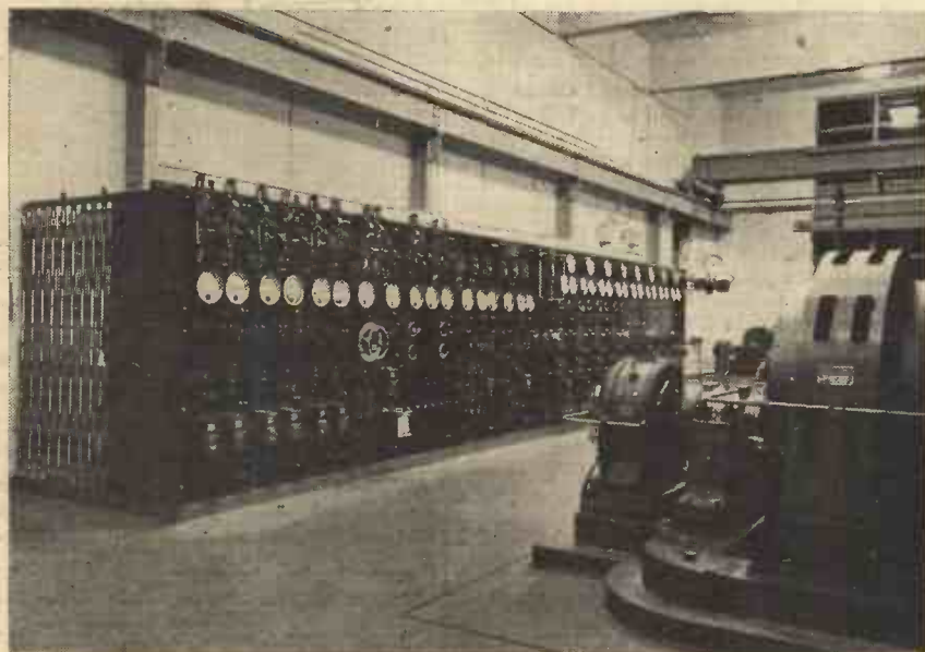
The switchboard and one of the generators.
